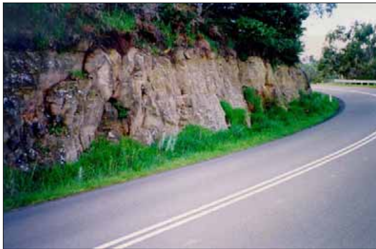
Figure 3: Table drain management at this site would minimise the risk of wildlife crossing for food and water. This is a high risk site because of the steep batter and sharp corner. (Zoë Magnus)
